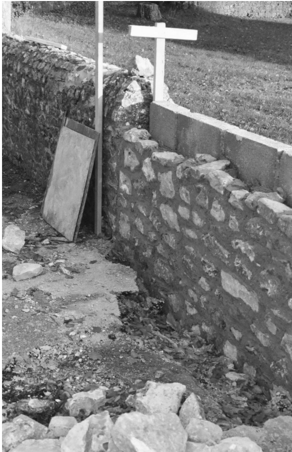
Figure 2 The need for skills in local materials. A good materials match, let down by excessive pointing in works to listed flint estate wall, Rousdon, Devon.
