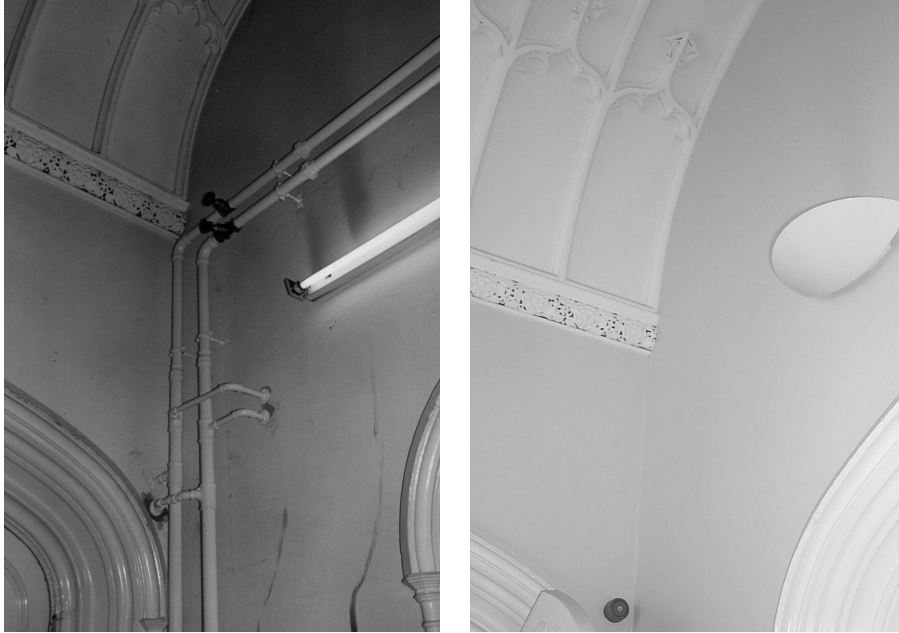
Figure 1 The need for awareness. New heating system and lighting in Grade I listed building, Kings College, Cambridge. The left illustration is as inserted by client and engineers without reference to architect. The right illustration is after remedial works designed and supervised by the architect. 1
